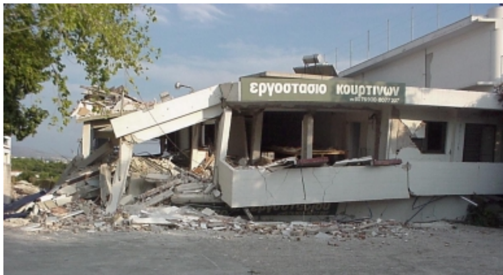
Figure 3 Location of Athens Earthquake , and typical damage ( http://www.itsak.gr/report.html )
