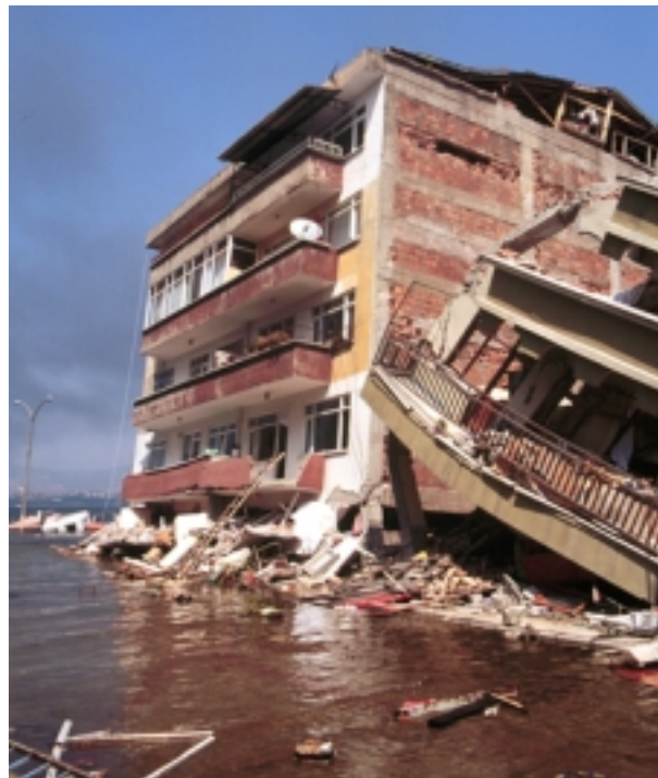
Figure 3 – examples of damage, Marmara Turkey earthquake.
